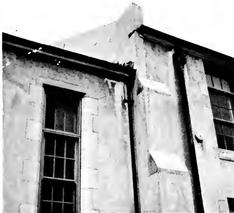
Photo 8. Morningside Elementary School. Pre-Field Act building. Parapet on verge of falling.
